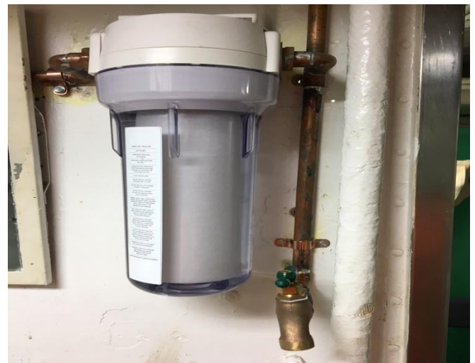
New filter installed by John Hudak
